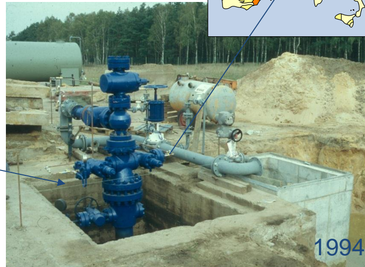
Head of reinjection well of geothermal DH system central in Neustadt-Glewe, Germany
